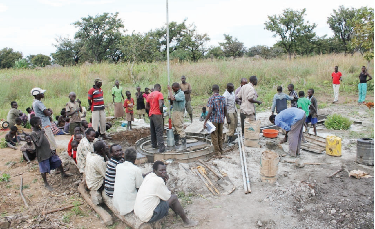
Casting and installation of a newly drilled borehole in Nabwal village, Napak.
