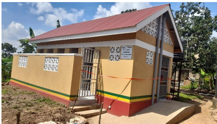
A waterborne toilet constructed by CIDI in Mugongo P/School in Kyengera Town Council
