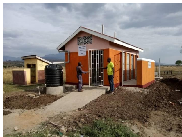
A VIP toilet constructed by CIDI at Nabulanger health center II in Loregae sub county Nakapiripirit District
