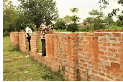
The headteacher Tubur primary school checking on the school dormitory under construction. Due to the uptake of school feeding by parents, they went ahead to contribute money to construct a school dormitory so that their children can learn fully.
