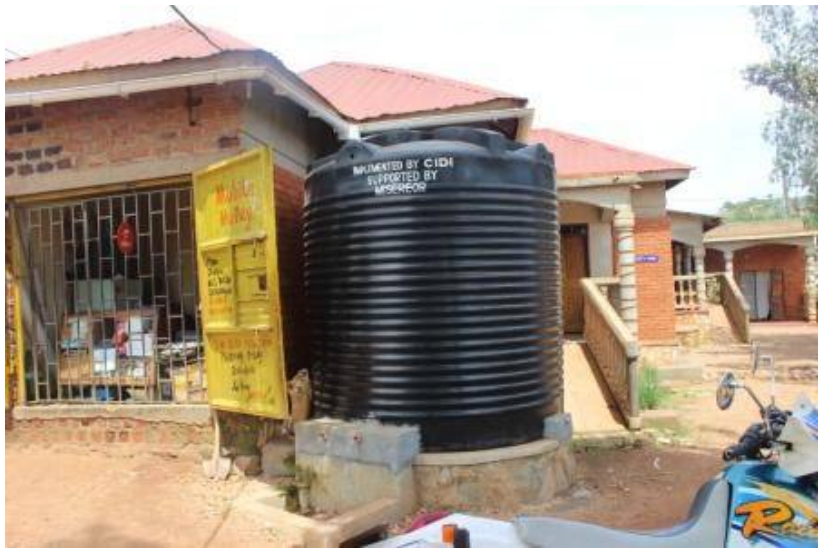
Rain water harvesting tank provided for communities in Kampala
