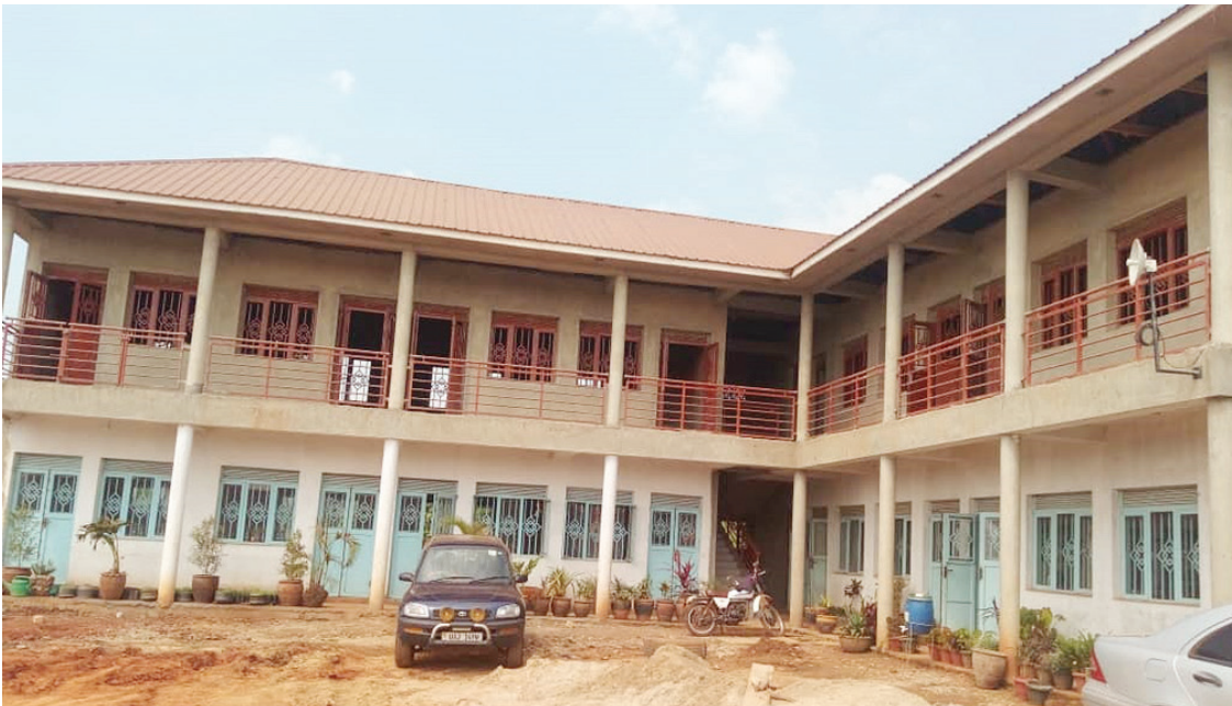
The CIDU Training Center for Gardening and Landscaping under construction with classes and administration block.
